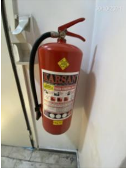
fire fighting equipment .JPG
