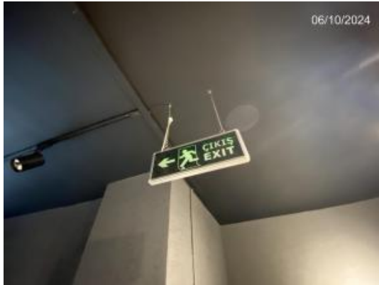
emergency exit sign .JPG
